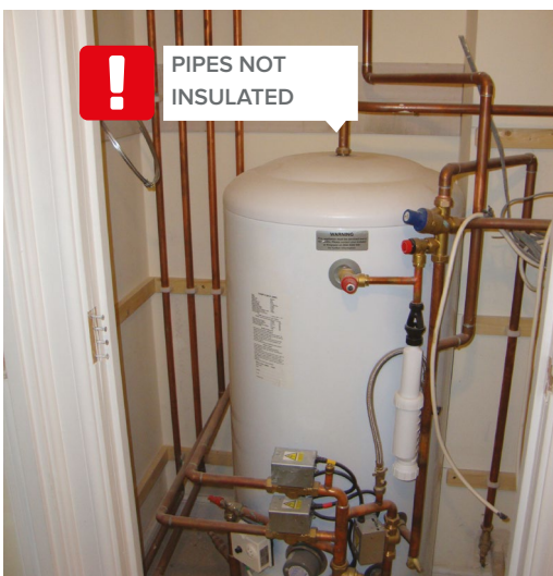
PRIMARY PIPEWORK NOT INSULATED
